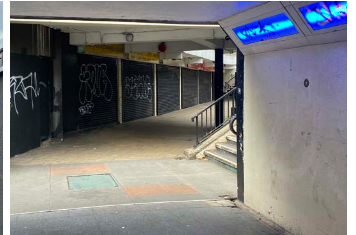
Subway ends in area with limited inter-visibility
